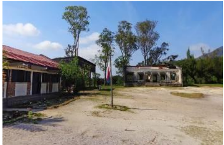
View of the Mahatalaky EPP school complex before the new building. From left: functioning classrooms; ruined building; building in need of repair (lefthand classroom still in use); site of new building
