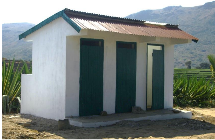
Newly constructed latrine blocks at Mandiso Lower Secondary School with handwashing stations and MHM facilities.
