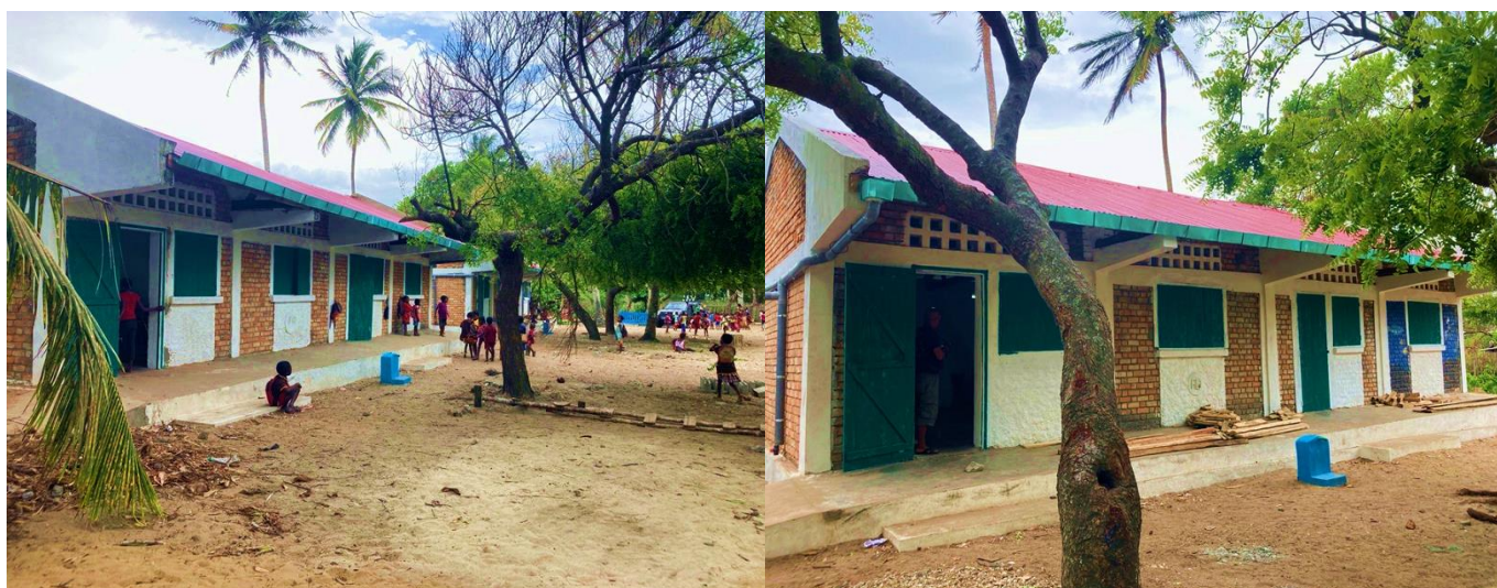
New timber apex frames and metal sheet roofing has been installed on both existing school buildings at Sainte Luce Primary School.
