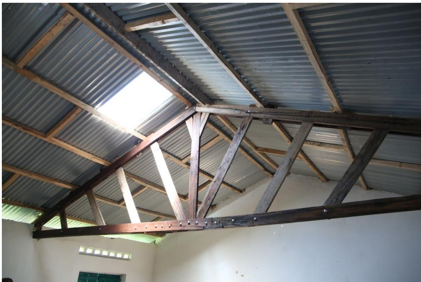
Refurbishment of the roofs of both school buildings were completed in December 2022.
