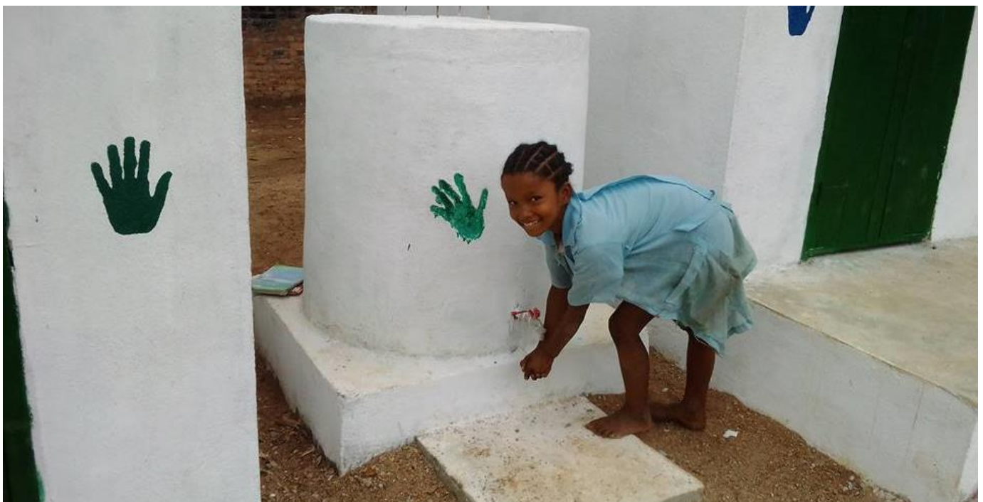
A student washes their hands using the newly-installed taps connected to a piped water source
