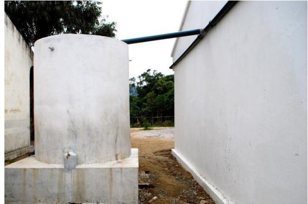
The completed rainwater harvesting system
