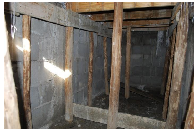
Scaffolding is used inside the latrine pits to support the construction of cubicles on top
