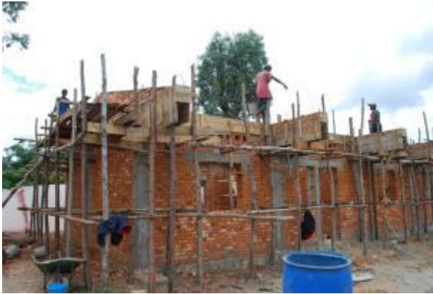
Brick laying finished and pillars, lintels and eaves over windows filled with concrete
