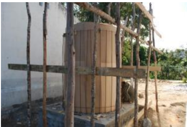
Wooden mould for the rainwater harvesting tank's walls erected inside the wire reinforcement cage
