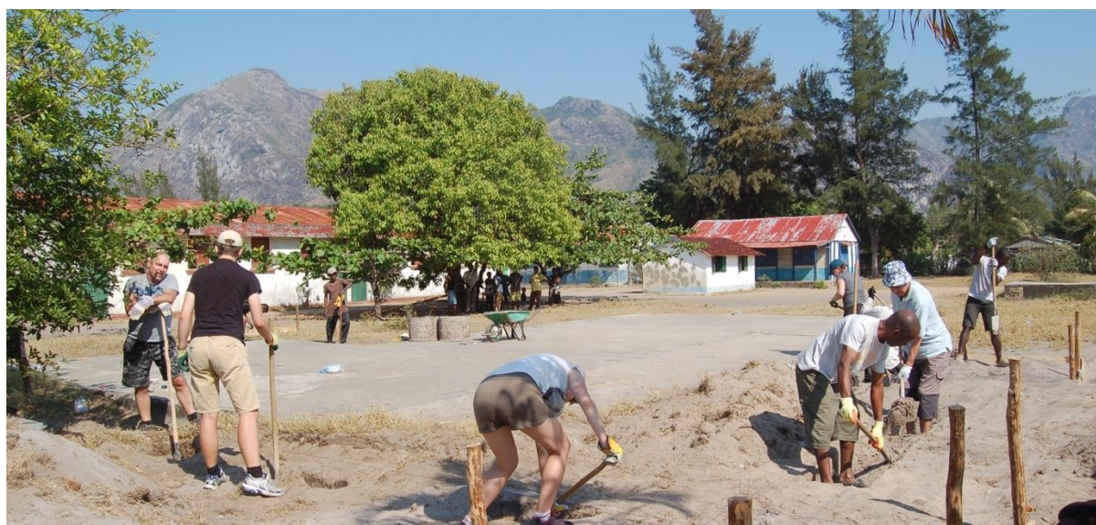
Community Development volunteers and SEED's construction team digging the foundations at Lanirano Primary School in September
