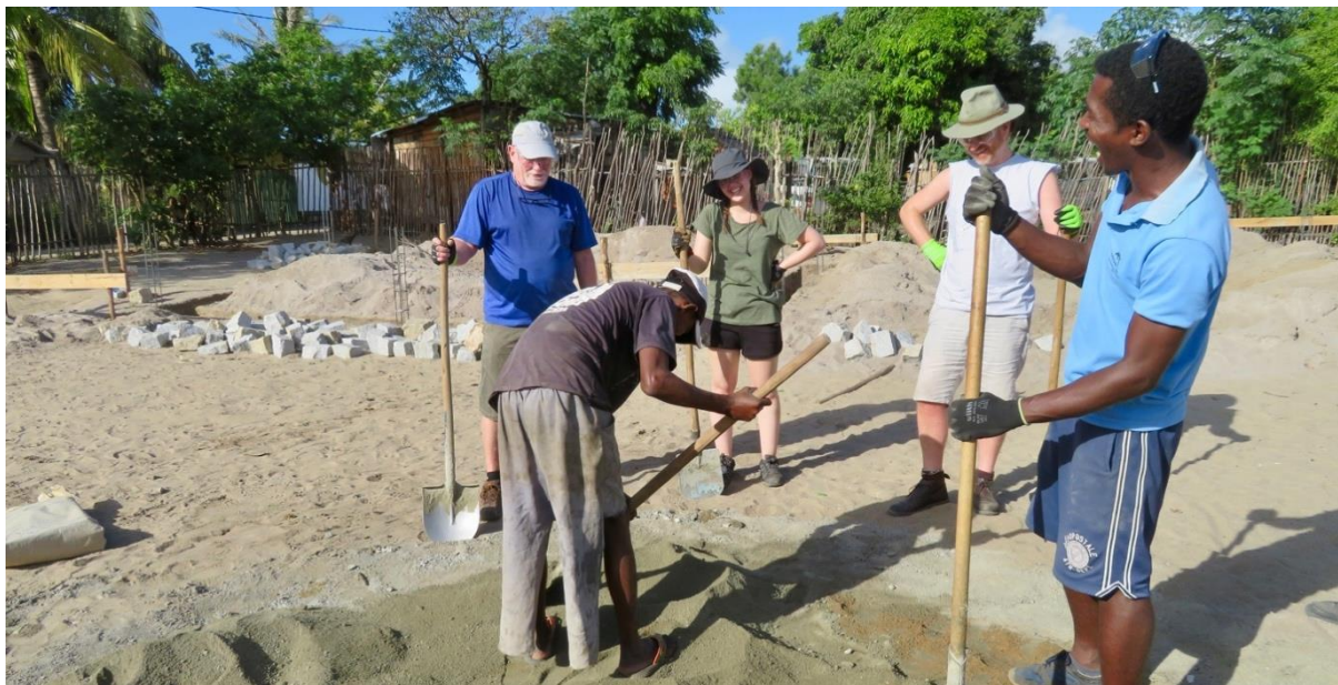
Community Development volunteers have been working alongside SEED's experienced construction team in Manambaro
