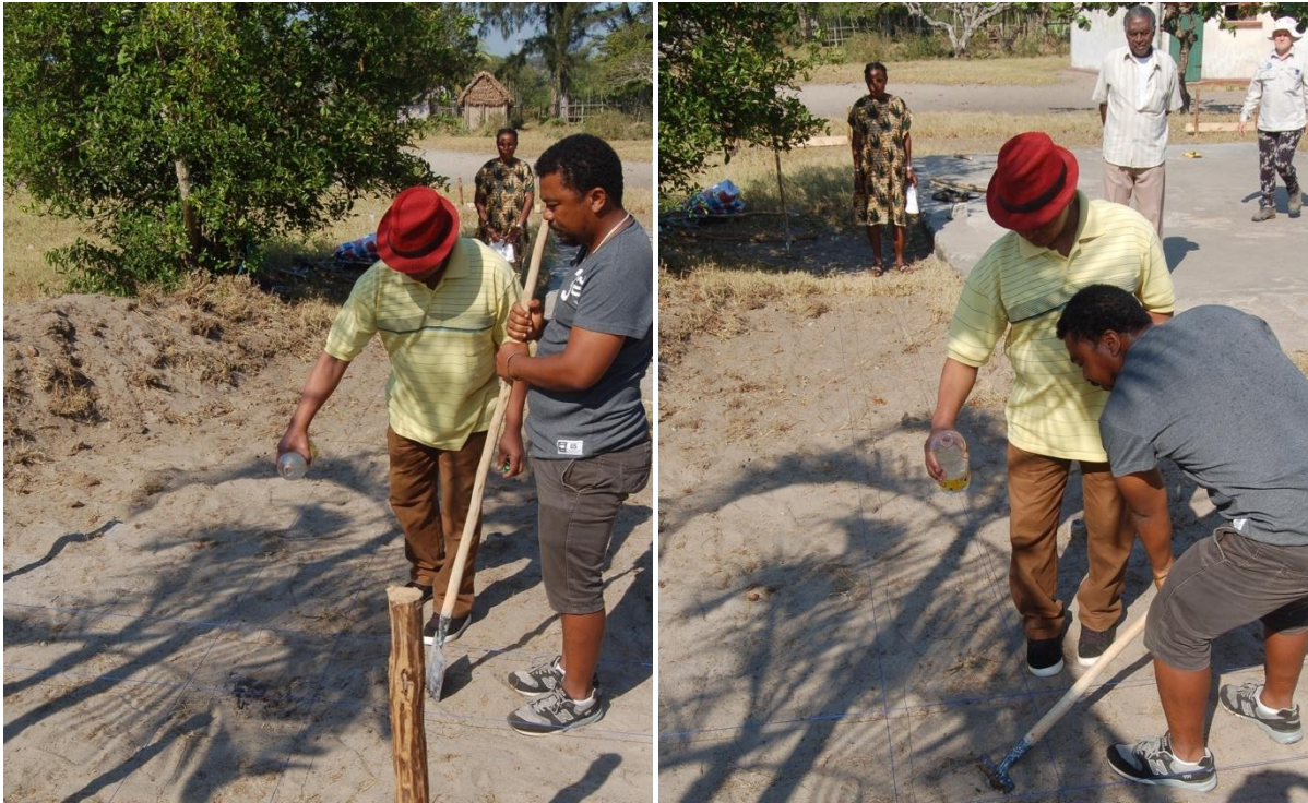
Lomba, SEED's Head of Construction, and the Chef fokontany of Lanirano leading the ground-breaking ceremony in late August
